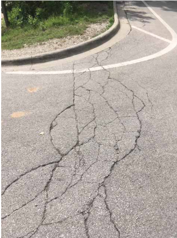
Movement in Roadway
