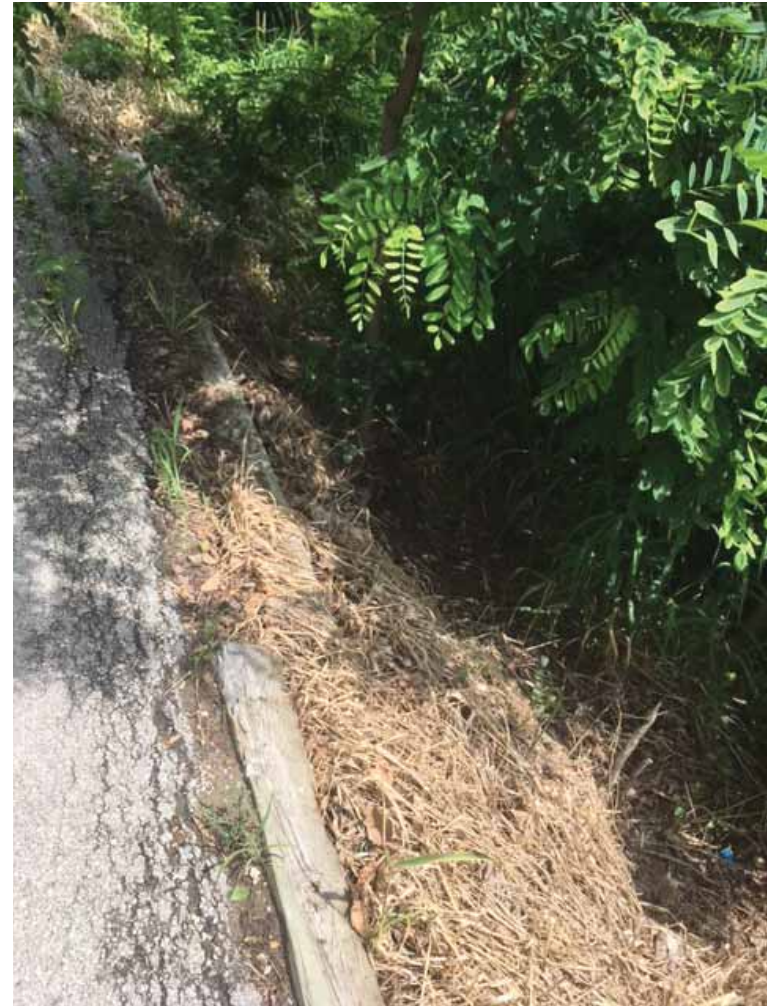
Edging/retaining wall giving way
